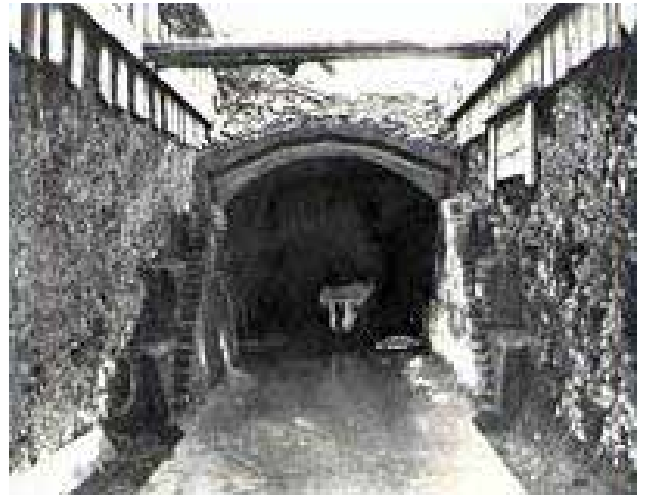
Cut and cover section of the aqueduct (1898) Courtesy of Powys Digital History Project
